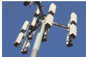
OUTDOOR WI-FI ACCESS POINT
